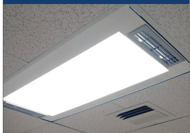
FIGURE 2. UV-C unit installed
